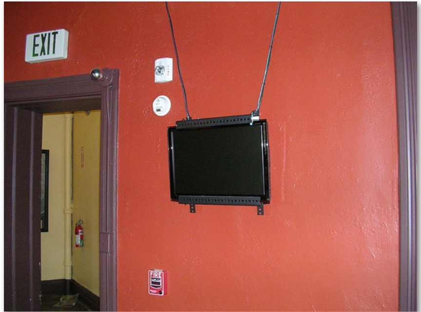
The two 24-inch monitors, power and data lines are suspended by cables from the dome sill retainers.
